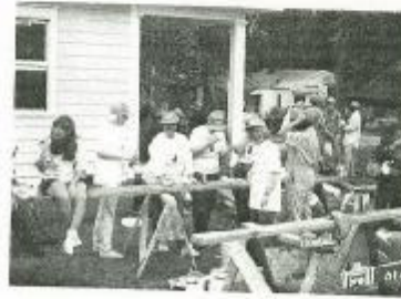
"Peachtree Lions Club of North Atlanta for its World Service Day project are shown working on a house being built by Habitat for Humanity."
